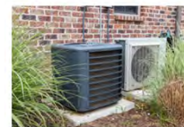
Photo of HVAC units.
